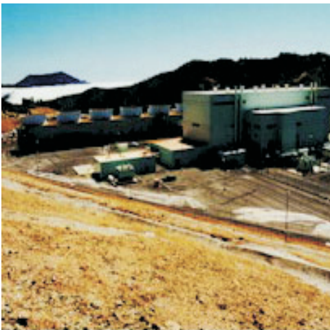
NCPA Geysers Power Plant
